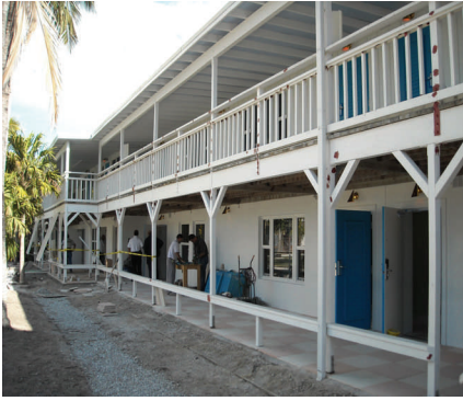
Naples Beach Hotel Architect: BSSW Architects, Inc. Old Florida "A" Building Renovation
